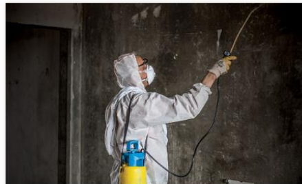
FIRE & SMOKE DAMAGE
