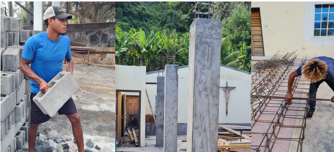
The rebuilding continues with work in preparation for the construction of a new roof on the Church building in Sandy Bay.
