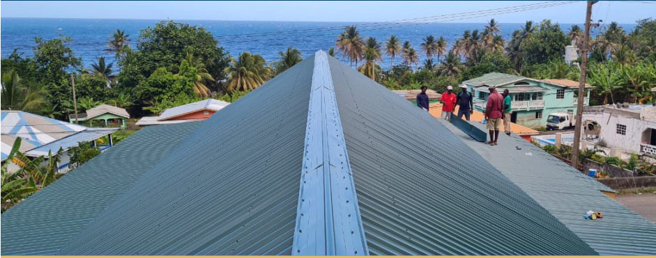
Through the generosity of many, a new roof was built in time for Easter!
